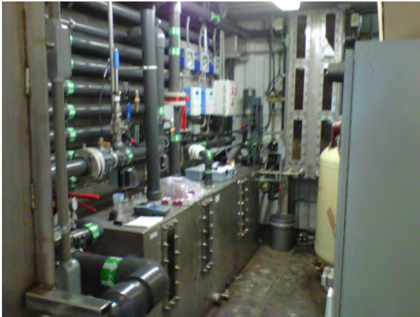
Figure 18: Krofta Sand Filter at ADM pilot plat
