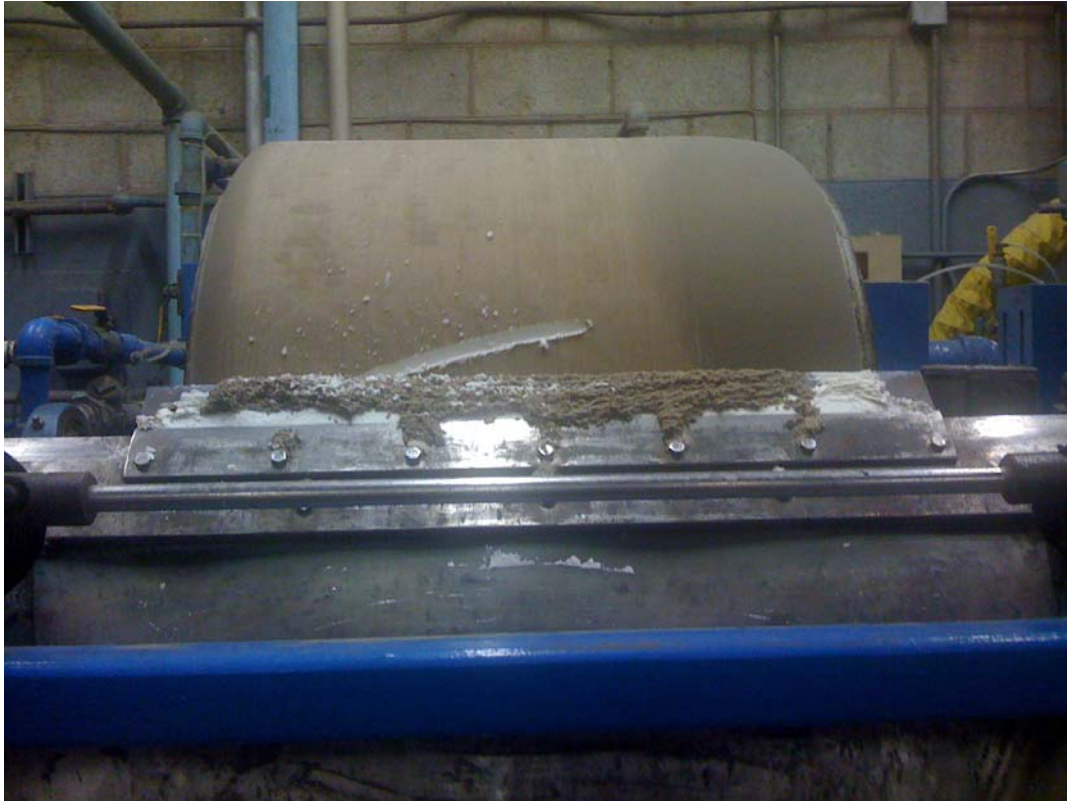
Figure 20: Alar RVF Filtration with FW40 precoat filteraid
